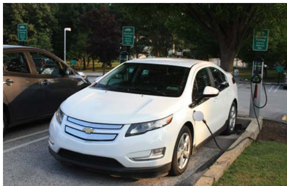
Example of an electric vehicle charging station.
